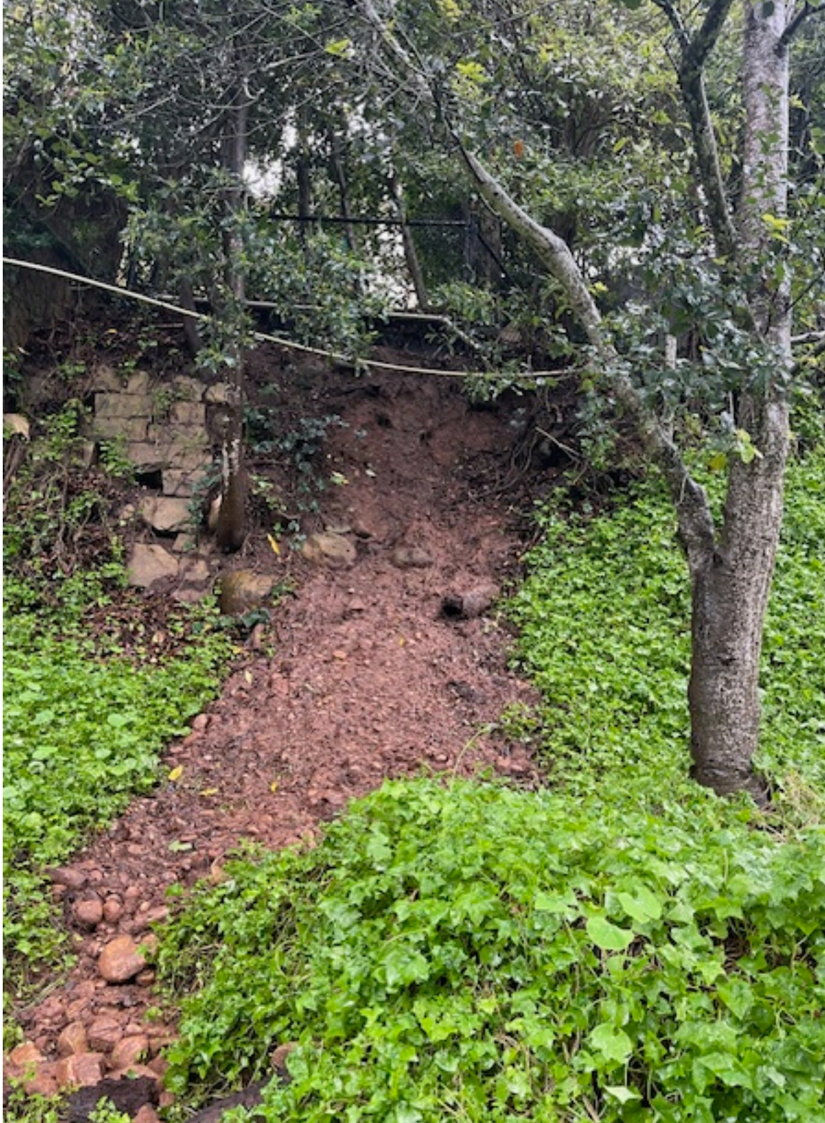
Photo 4 – February 2024 Slope Failure on East Embankment
