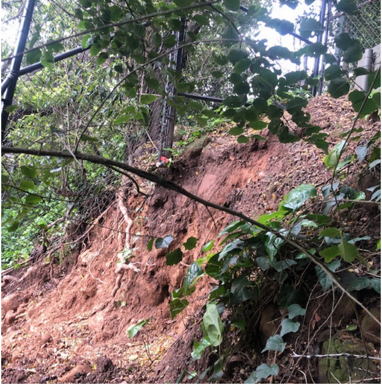
Photo 2 – Looking South Showing Slope Failure on East Facing Slope/Embankment from January 9, 2023 Historic Rain Event.
