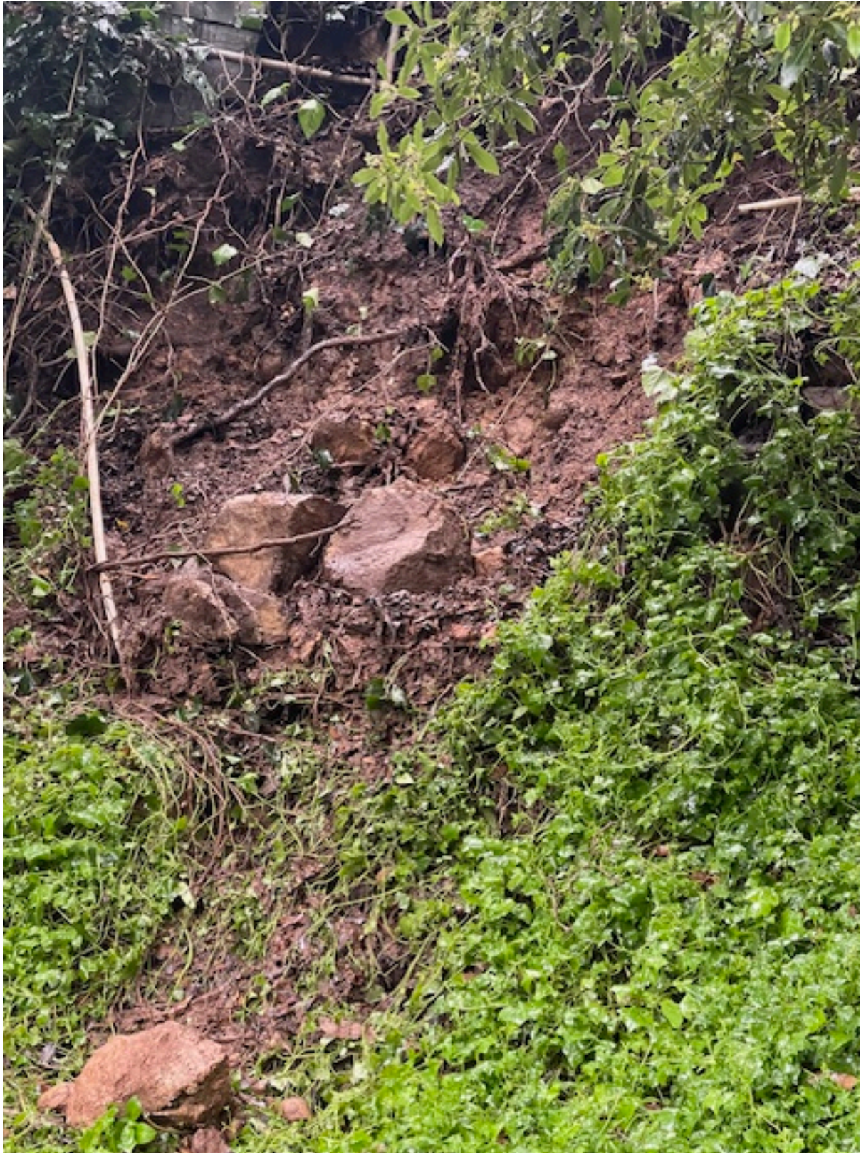
Photo 3 – February 2024 Slope Failure on East Embankment
