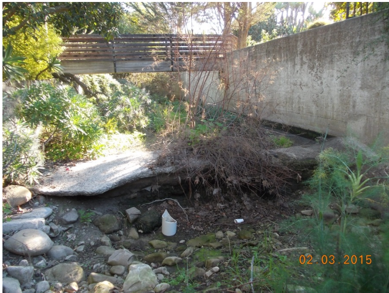
c. Channel upstream of bridge, note exposed pipe encasement
