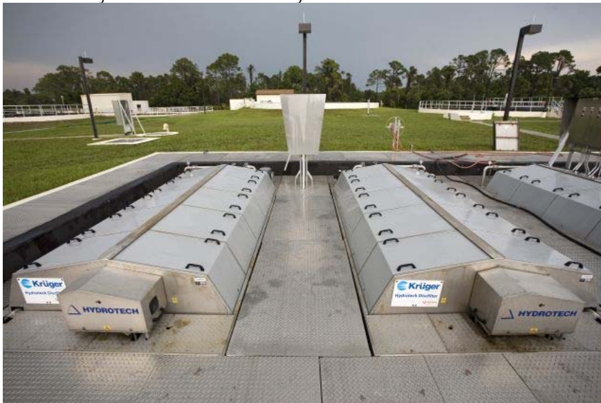
FIGURE 3-7 A Full-Scale Hydrotech Disc Filtration Facility
