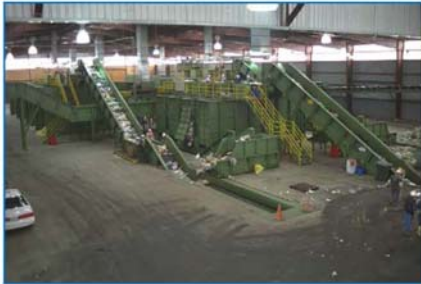
Kings County, CA – Mixed MSW Dirty MRF sorting system constructed in 1997
