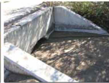
Drainage Channel Filled with Hillside Silt
