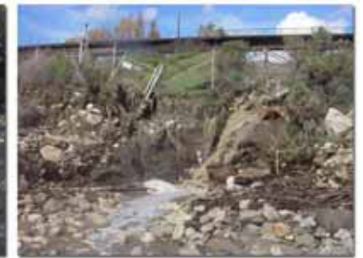
Erosion and Property Damage Caused by Runoff
