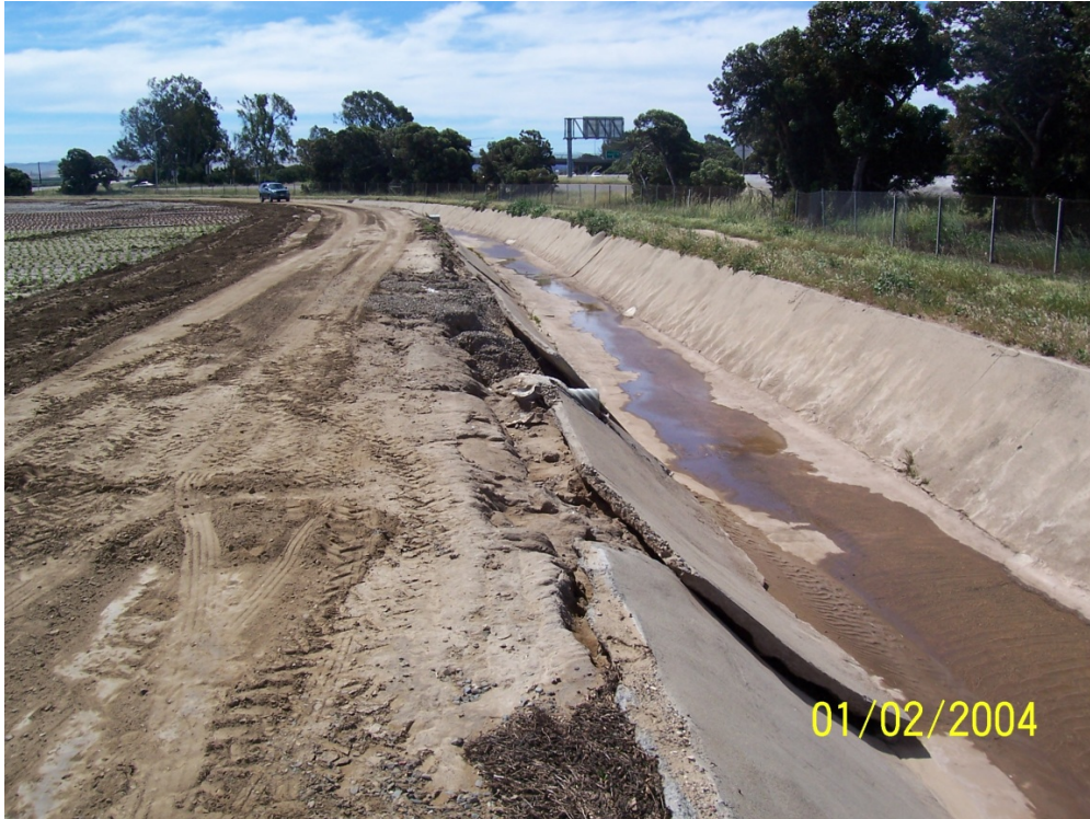
A portion of the concrete lined Bradley Channel in need of repair
