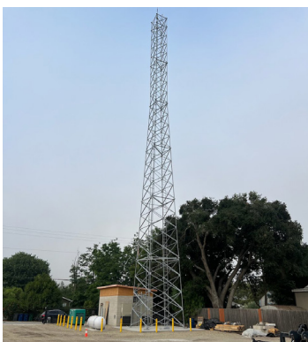
← Fire Station 24 Los Alamos 125’ tower, a Turner & Townsend Heery project for the County of Santa Barbara
