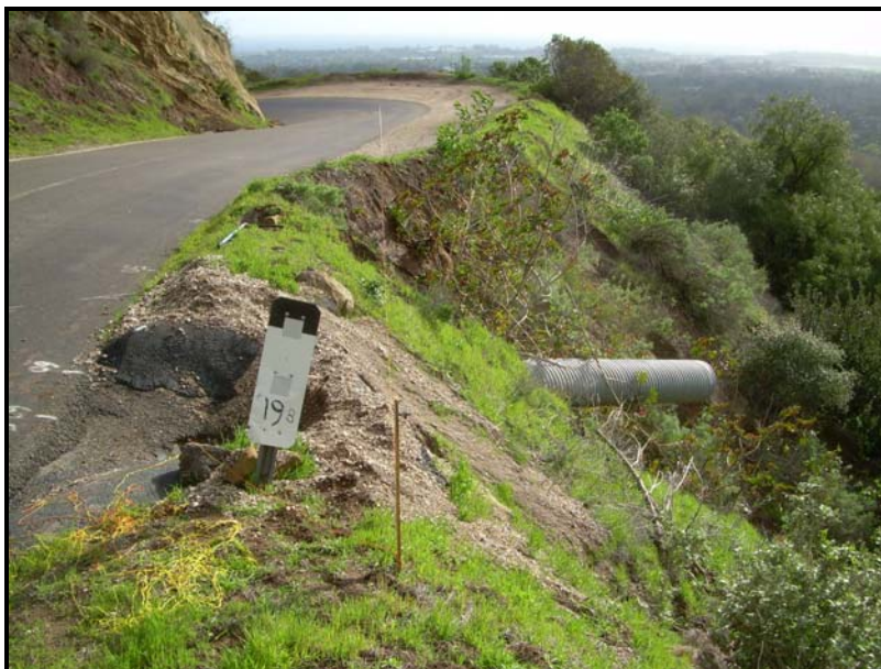
Figure 2: Failed slope on San Marcos Road at Mile Post 1.7.
