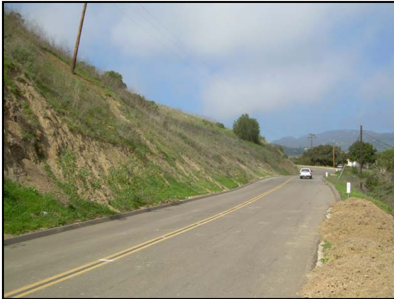
Figure 1: Eroded slopes on San Marcos Road at Mile Post 0.7.
