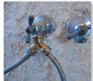
Modern laundry detergents work fine in cold water. Turn off the hot water supply to your washer and reduce your water carbon footprint significantly. With a wye supplying cold water to both the hot and cold inlets, the washer will not stall if someone selects hot water.
