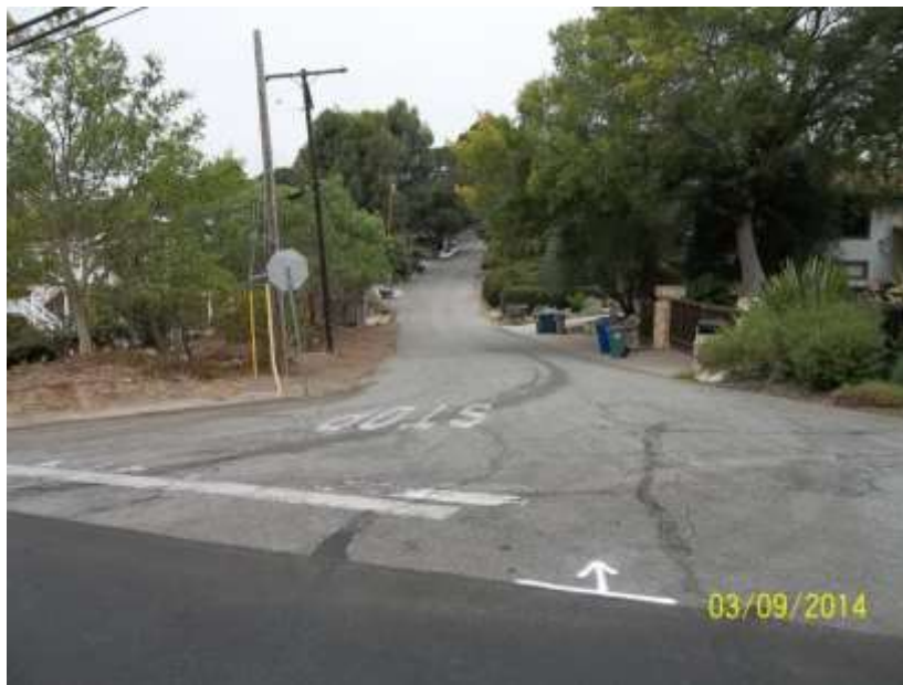
Typical road to be resurfaced on Ben Lomond Dr.
