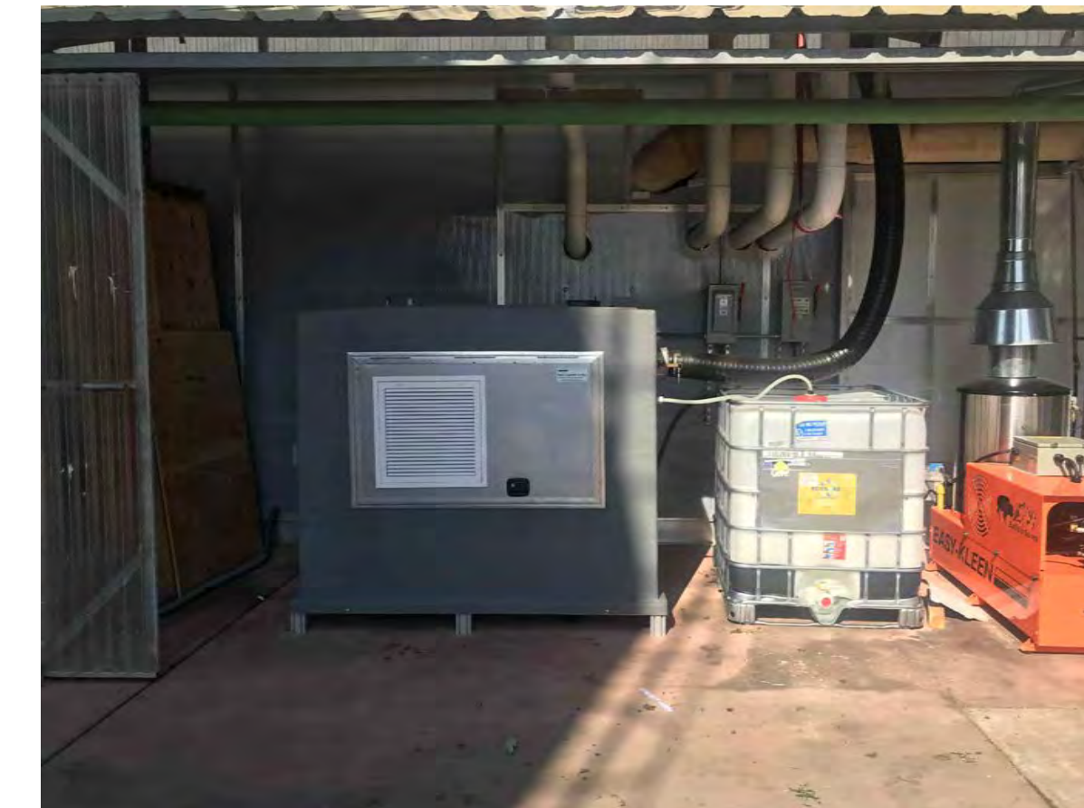
ODOR CONTROL UNIT 2
