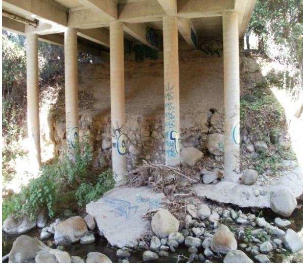
Western side Toro Creek bank
