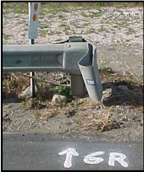
Photo: Damaged Wrap Terminal
