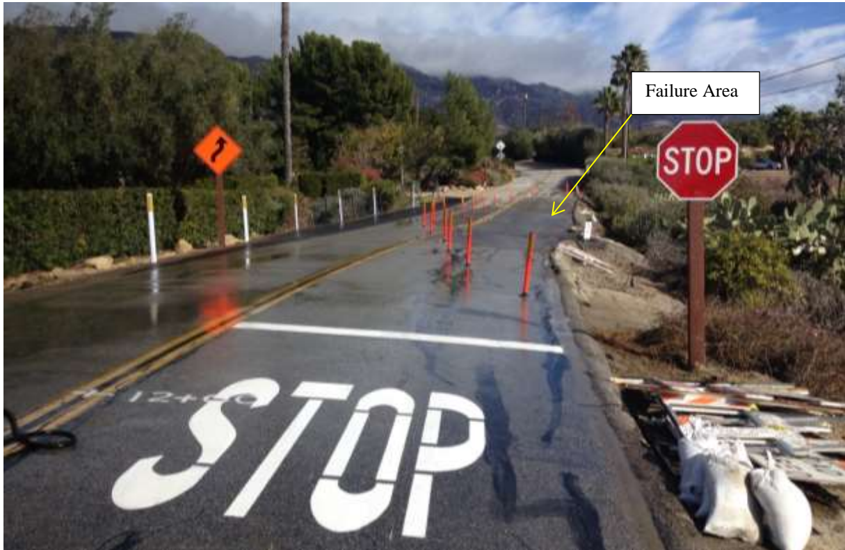
View of Ortega Ridge Road, looking east, showing temporary traffic controls. Area of roadway that is delineated by orange channelizers continues to differentially settle, and has continued into left-hand lane.
