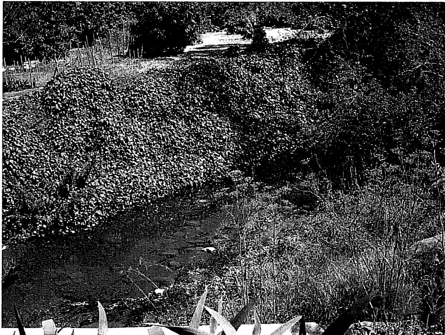
Debris Rack location.
