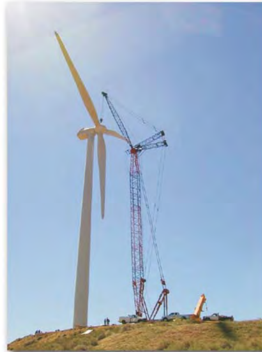
Inset E: Typical WTG construction. The WTG is a 1.5-MW machine. (Photo Credit: Michael D. Burns, Oak Creek Energy Systems Inc., Mojave, California.)
