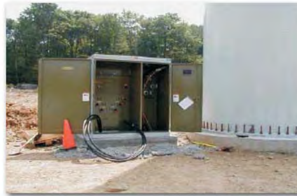
Inset B: Pad transformer beside WTG.
