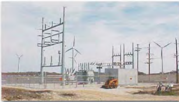
Inset D: Substation and interconnection facilities.
