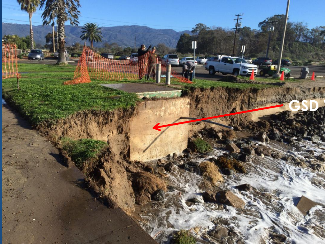
Wave erosion exposed Goleta Sanitary sewer outfall vault
