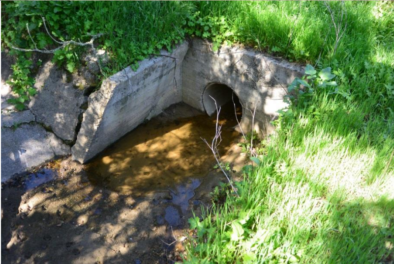
Photo 29. Crossing #3: 24-in. RCP culvert outlet structure that conveys water from man-made drainage system (Class IV watercourse) underneath gravel access road and gravel pad. (photo taken 3/26/2019)
