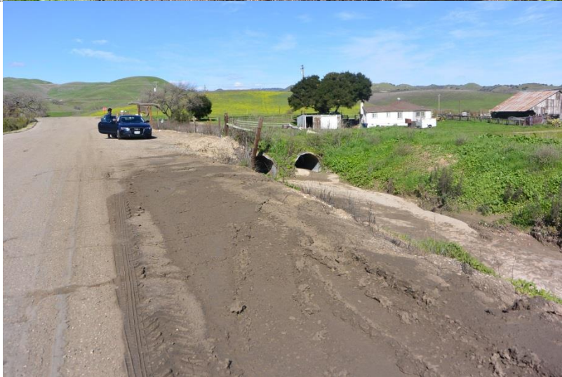
Photo 24. Crossing #1: Two 48-in. CMP (corrugated metal pipe) culverts at entrance to property near Highway 246. (photo taken 2/7/2019)
