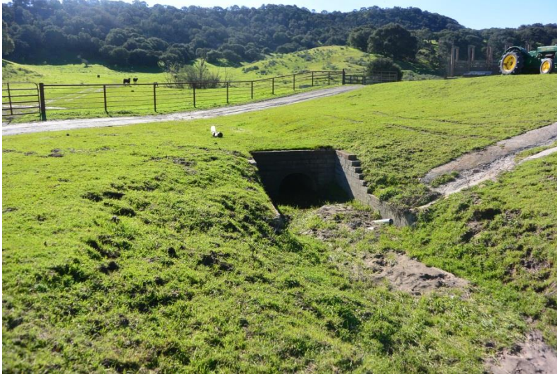
Photo 40. Crossing #2: 24-in. RCP culvert near proposed 2.55-acre cannabis premises area, which conveys water from man-made drainage system (Class IV watercourse) underneath gravel access road. (photo taken 2/7/2019)
