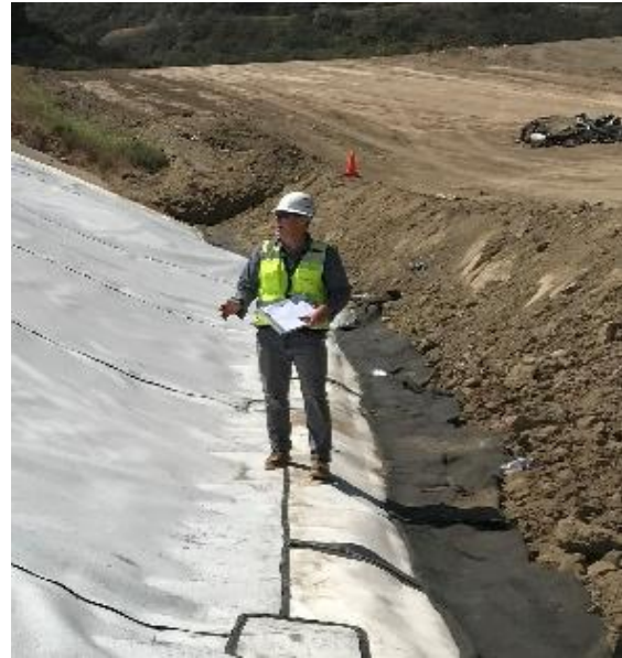
Geosyntec's CQA Monitor documenting geosynthetic repairs during construction of Tajiguas Phase III C Groundwater Protection System.
