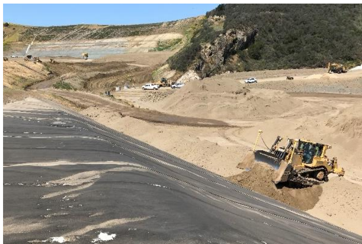
A dozer pushing protective cover soil up a lined slope at Tajiguas Landfill.
