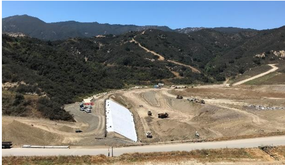
Geomembrane placed along an engineered fill berm during construction of Phase IIIC.
