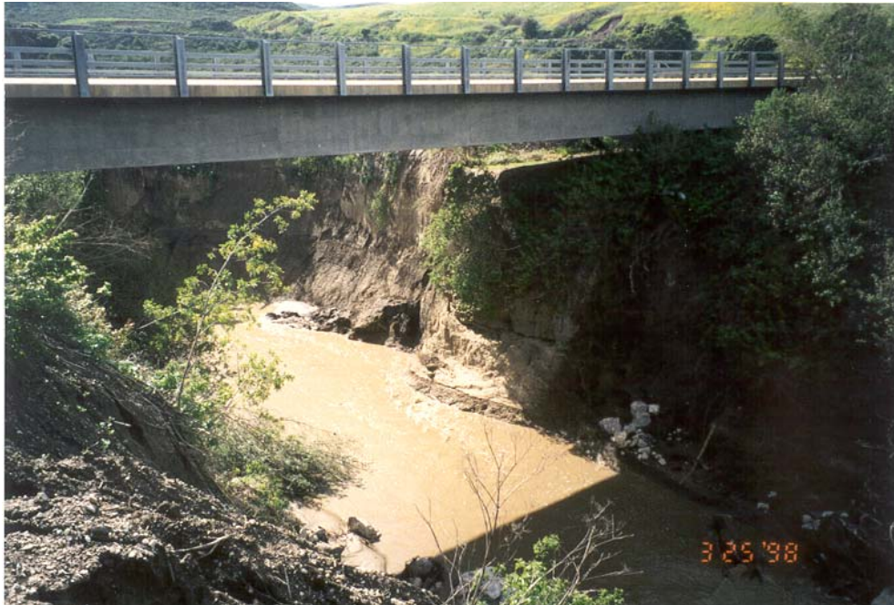
Photo: Existing Salsipuedes Creek embankment conditions at Santa Rosa Road Bridge 51C-020
