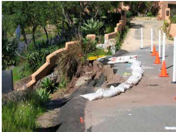
Photo: Post-storm Conditions at 584 Freehaven Drive (Site 1T68)
