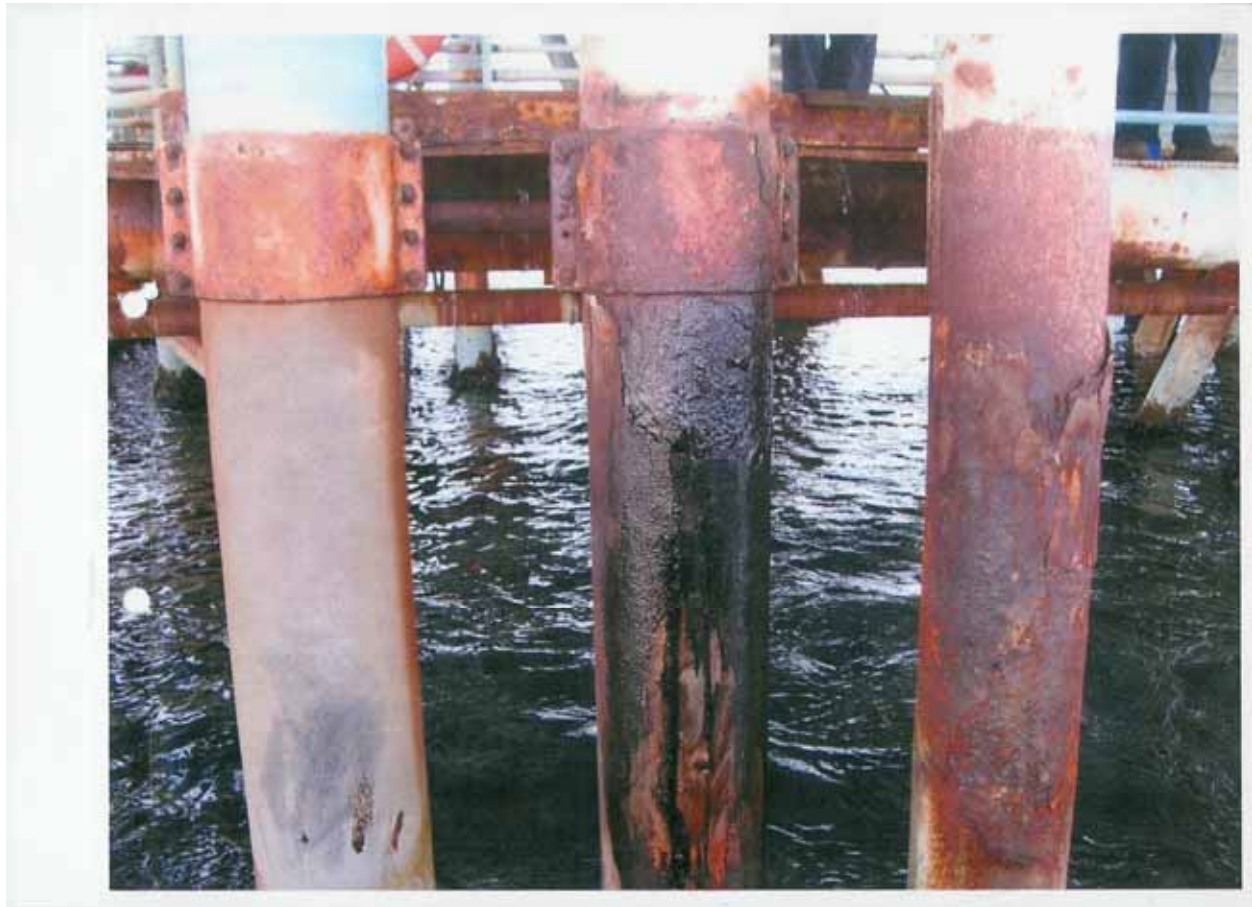
Figure 2: Some of the Shipping Pump Cans on Platform A, including the One that Spilled Oil on 12-07-08
