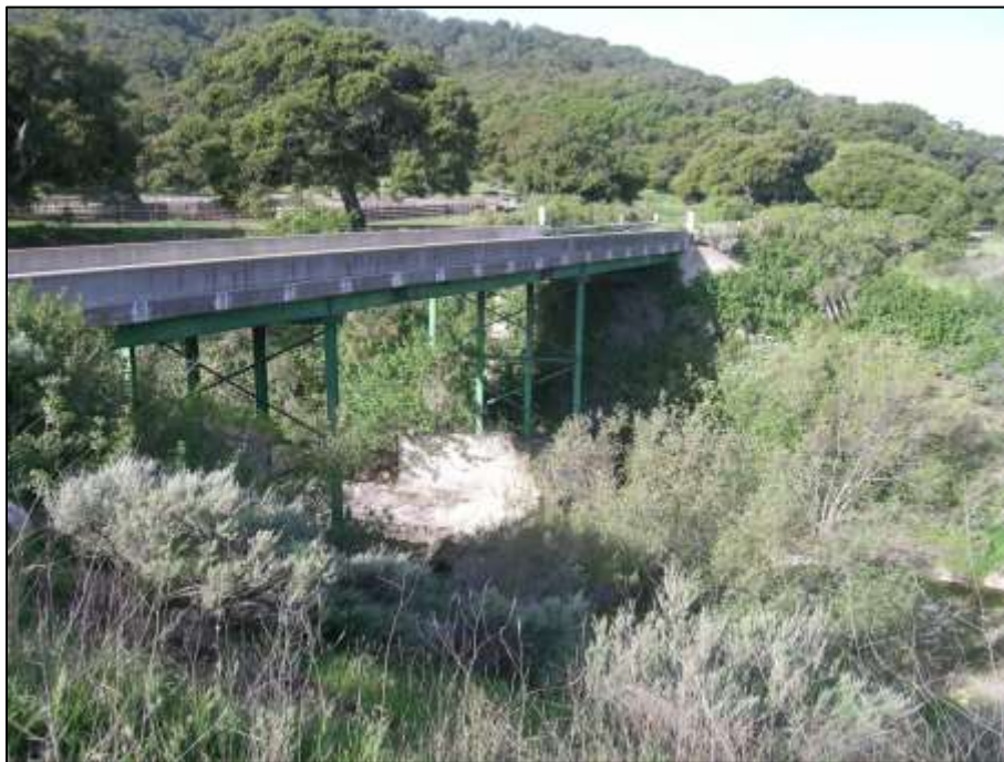
Existing Jalama Road Bridge No. 51C-0017 over Jalama Creek, looking upstream and to the Southwest.
