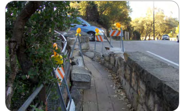
ACCIDENT DAMAGE TO MISSION CREEK BRIDGE
