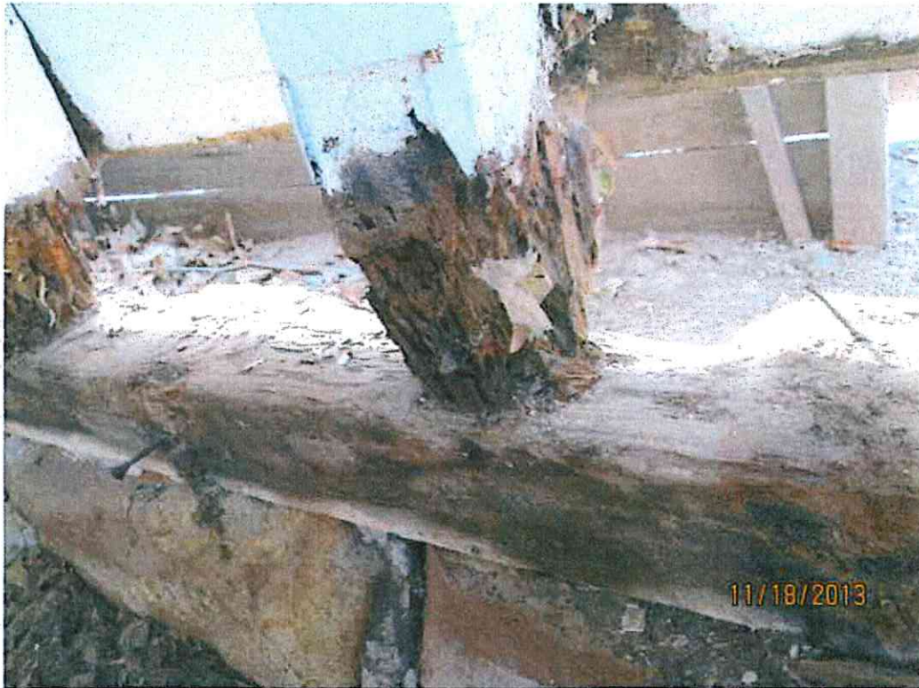
Plate 6. Deteriorated tower structural members resting on stone foundation. Photo: Danny Townsend
