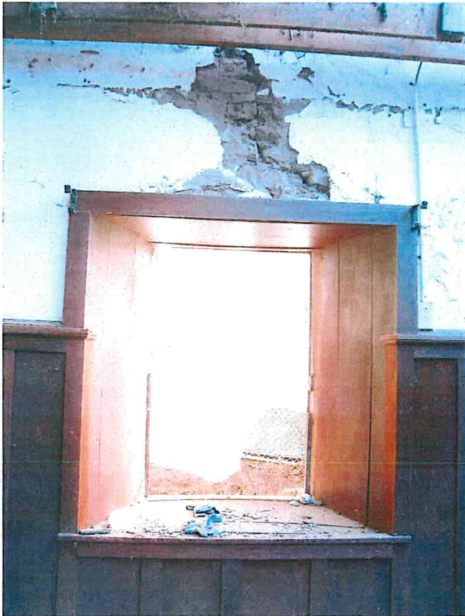
Plate 3. Adobe east wall showing structural cracks in adobe blocks
