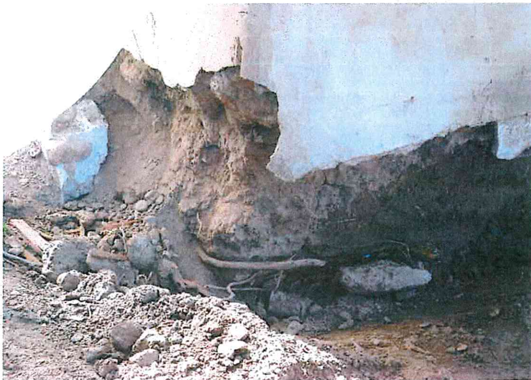
Plate 5. Detail of crumbling adobe blocks at base of northeast wall.
