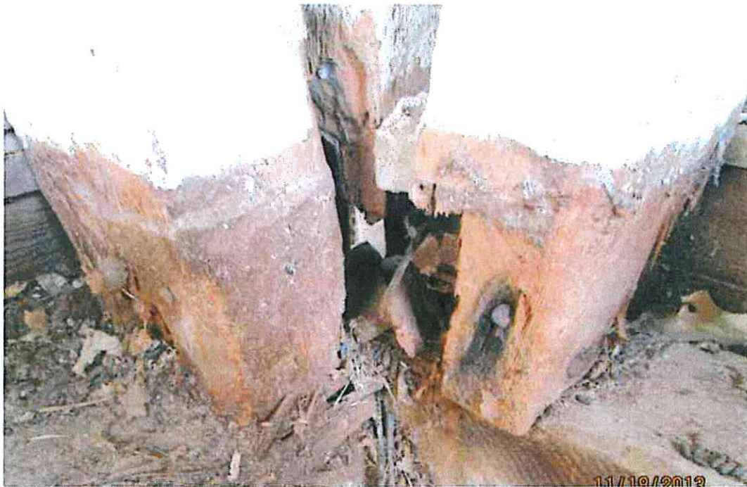
Plate 7. Deteriorated tower structural members. Photo: Danny Townsend
