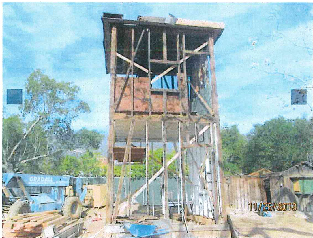
Plate 9. Tower showing deteriorated structural members.
