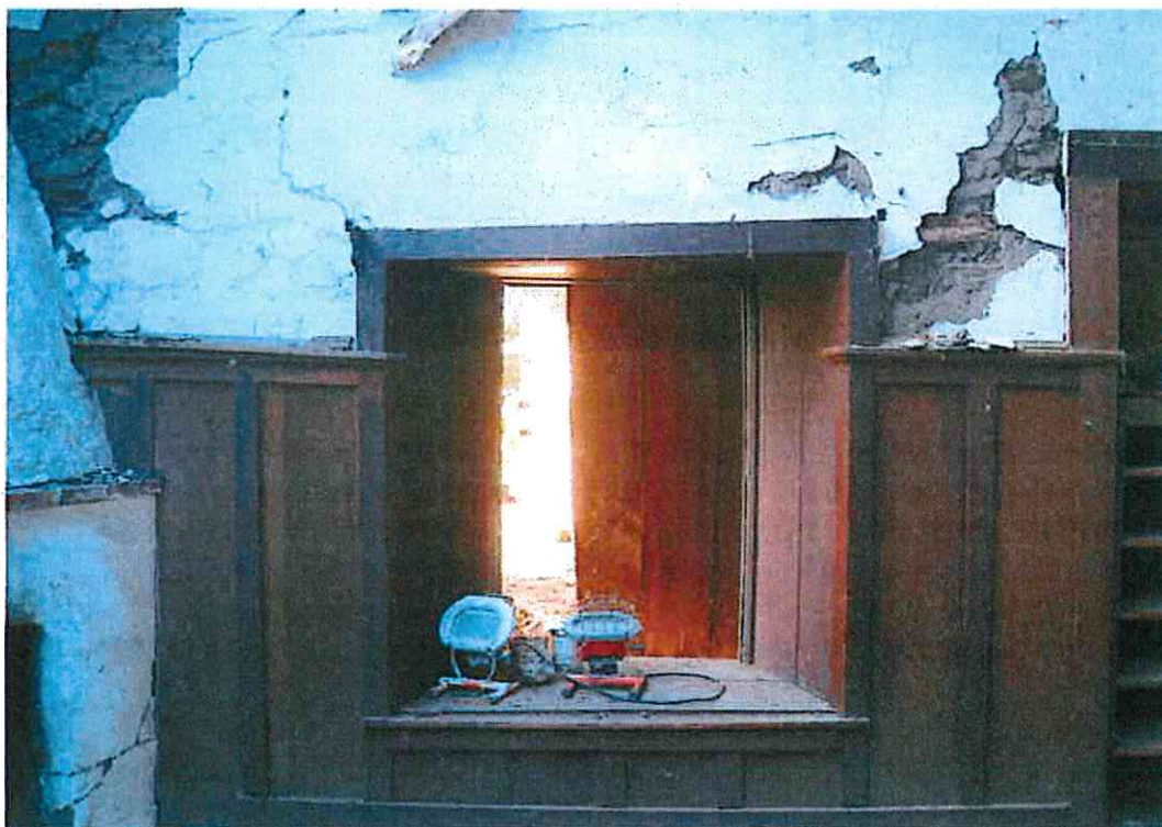
Plate 1. Adobe west wall showing deteriorated blocks.
