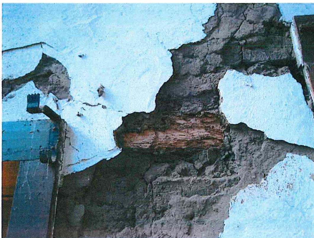
Plate 2. Detail of adobe west wall showing dry rot in structural wood member.
