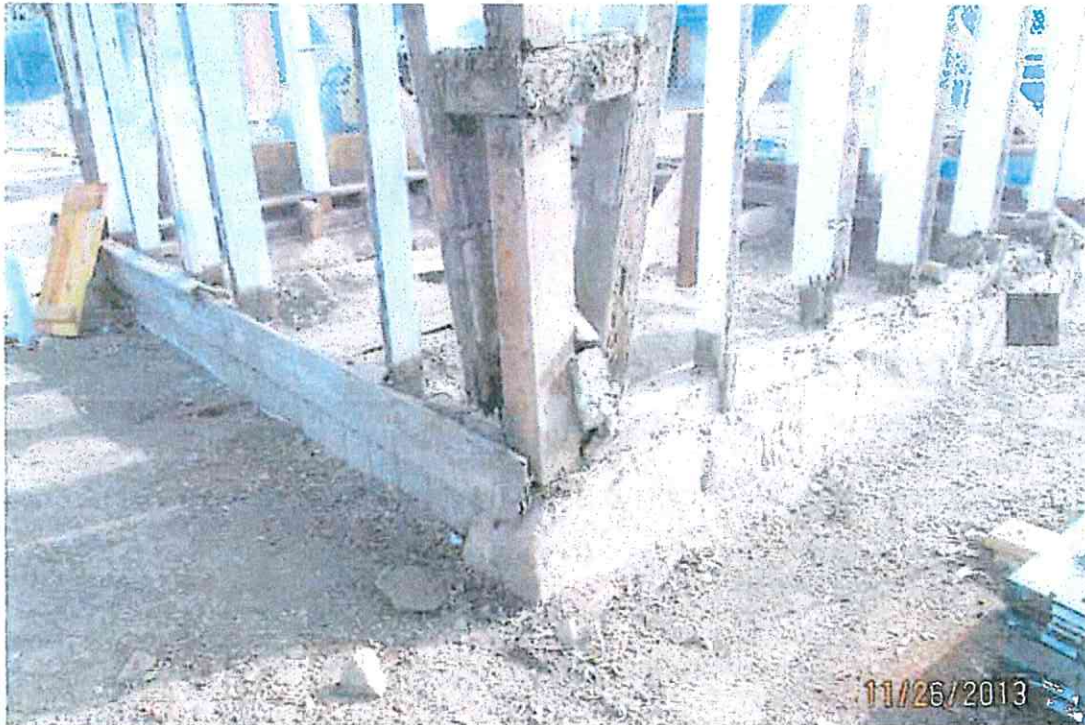
Plate 8. Deteriorated tower structural members. Photo: Danny Townsend
