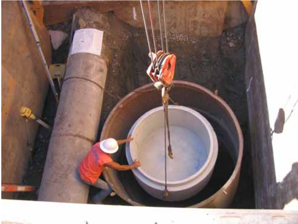
Installation of a CDS Unit at the Escondido Pass site in Isla Vista
