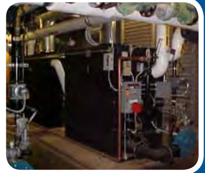
New high efficiency boilers in the County Mail Jail.
