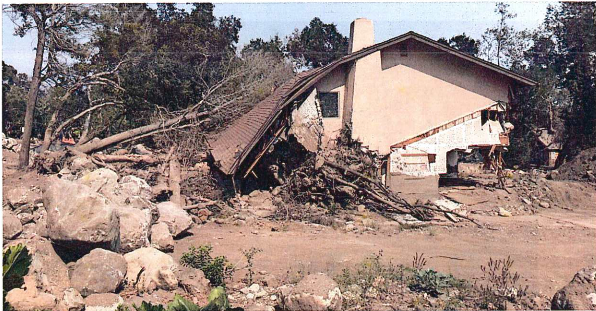
Figure 9. Destroyed home on San Ysidro Creek, located approximately 1 km from the fan apex. BGC photo, July 2018, looking east.
