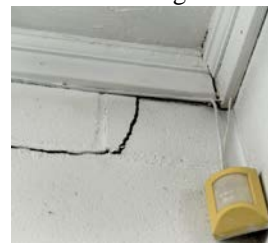
Plate 1: Cracks in a structure due to blast induced ground vibrations (Source: Google Images)
