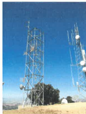
Facility 3 south – SBA Towers II
