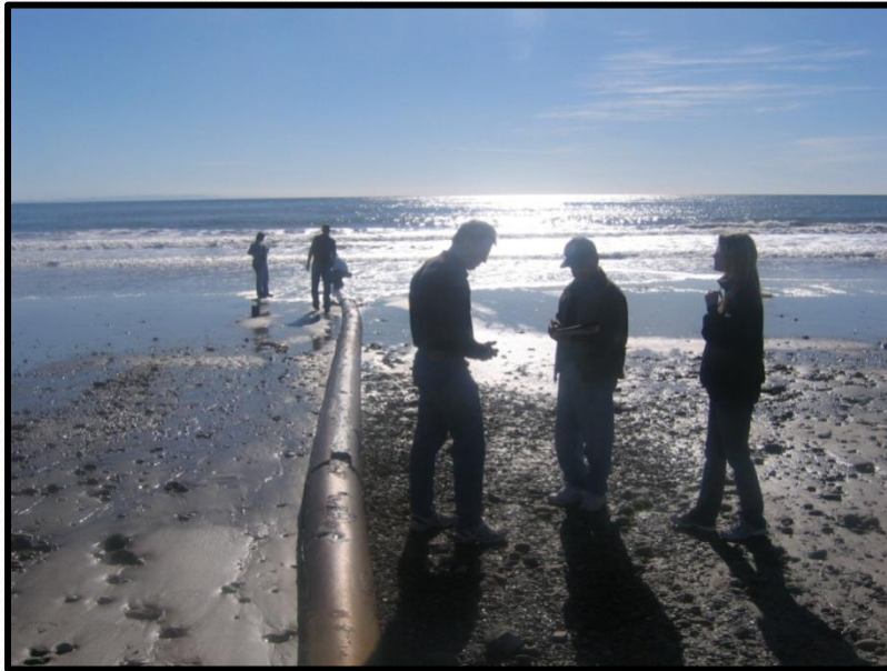
Site 4, 5/Ellwood Beach Pipeline Hazard (2008)
