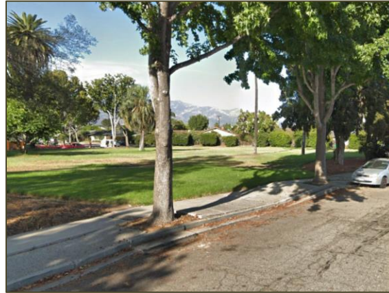
Typical Hardscape repair due to tree roots. San Juan Place- lifted and damaged sidewalk, curb and gutter. Pavement is also failing due to saturation from ponded water.
