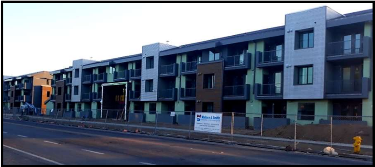
Picture of Residences at Depot St. during construction, photo provided by Prop 63 funded Help@Hand team
