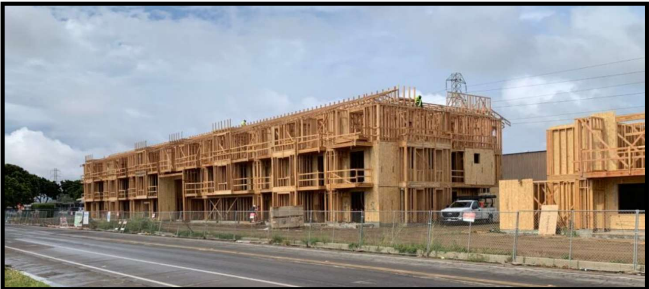
Picture of Residences at Depot St. during construction, photo provided by Housing Authority of County of Santa Barbara
