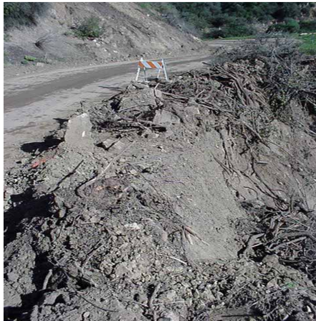
Photo: Post-storm Conditions at M.P. 0.8 (Site 1T32)
