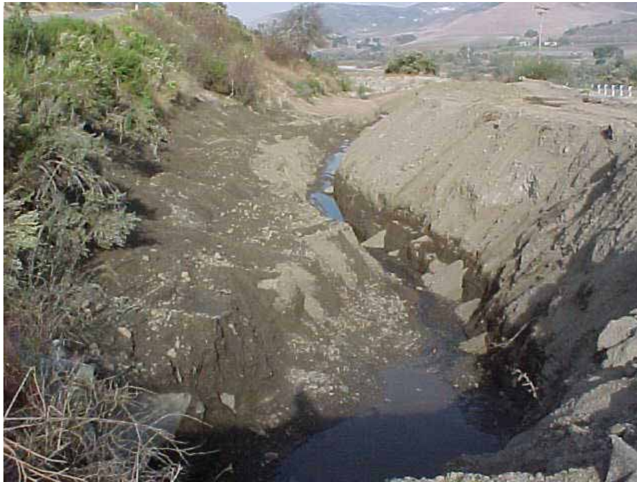
Channel Clearing North of Santa Rosa Road on Shale Creek Looking Northwest (downstream)
