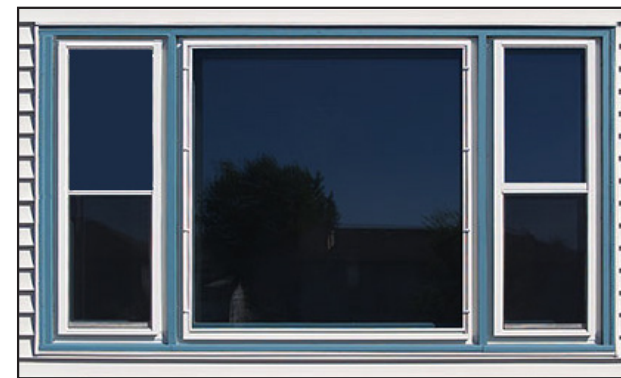
Figure 6.7 – Example of Inappropriate Window Relief and Dark Reflective Glazing
