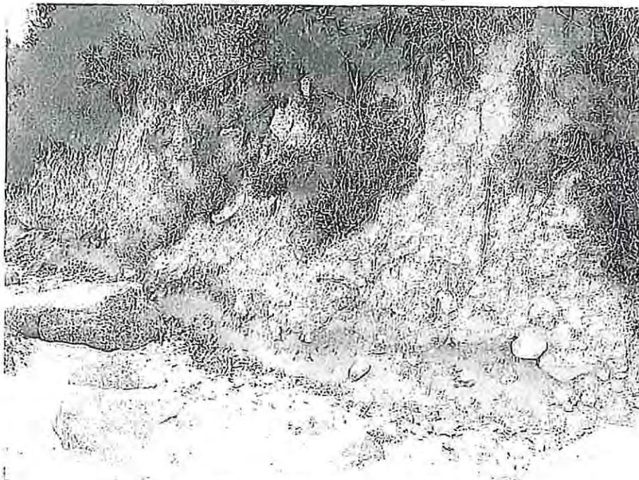
Photograph 8. Close-up of under-cut toe, bluff area below existing residence, and scattered rip-rap slope protection, viewed to northeast.
