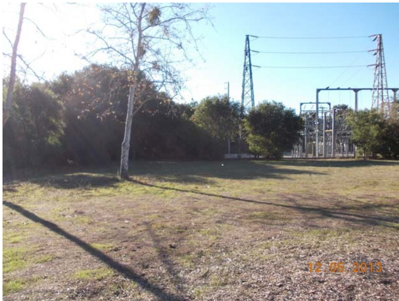
c. View of SCE substation from Kellogg Open Space
