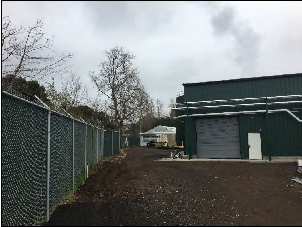
Photo 1: Greenhouse and broiler to be demolished in ESH Buffer (Aspect: East). Photo taken 2/27/2019.
