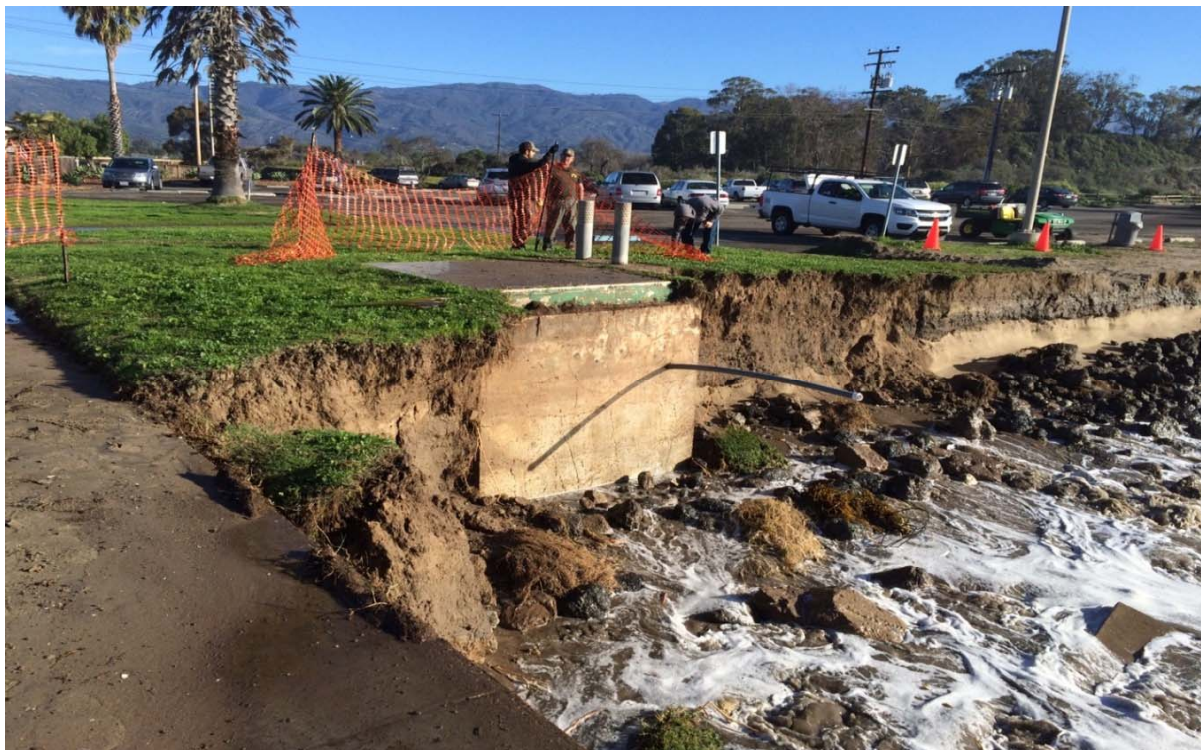
Photograph I. Exposed Face of Goleta Outfall Vault and Cathodic Protection Facilities
