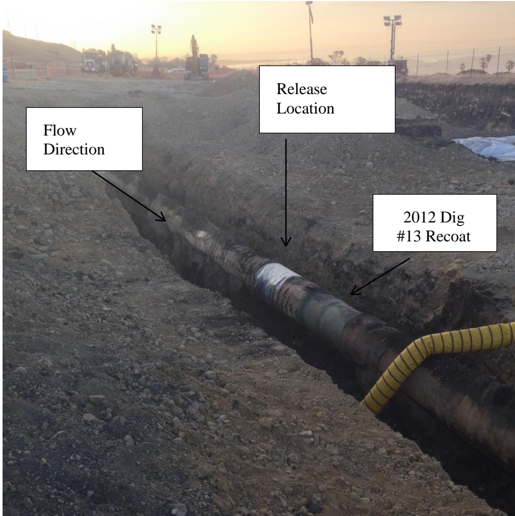
This picture shows the release site wrapped in plastic 6 feet upstream from girth weld 5940 where the coating repair is visible. The repair was identified as Dig #13 from the Post 2012 ILI Survey Anomaly Digs.
