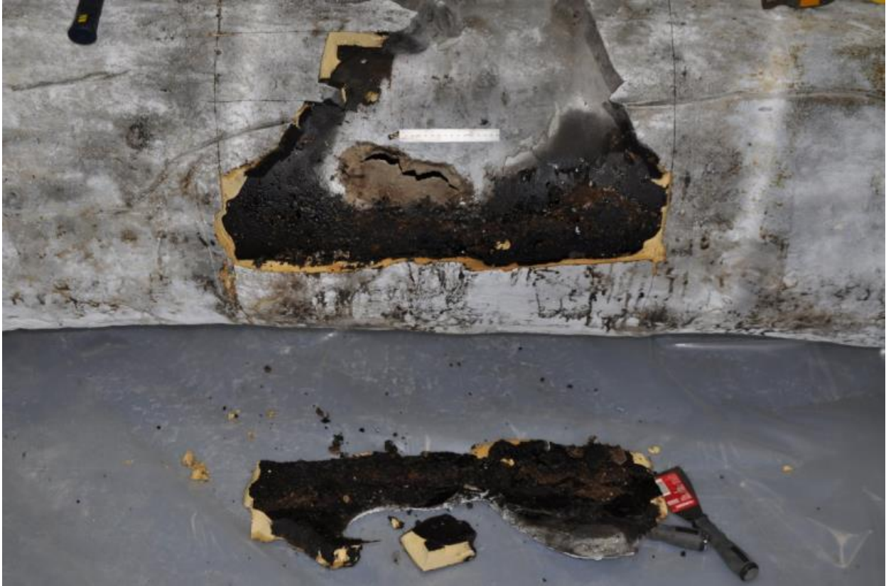
This picture is excerpted from the final metallurgical report. “Figure 16. Photograph showing a piece of insulation removed from adjacent to the failure location; near 4:30 orientation.”
