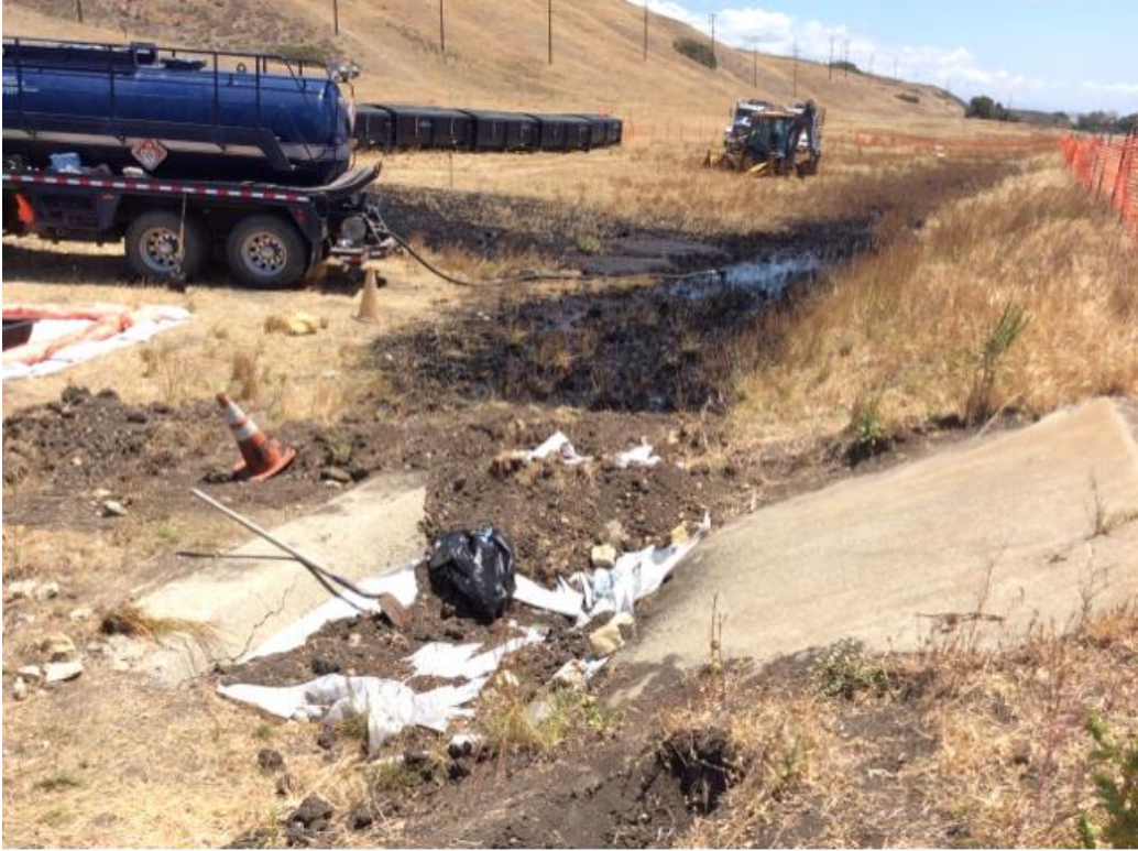
Release Site with Culvert in the foreground. Vacuum Truck sucking up pooled oil in the background.
