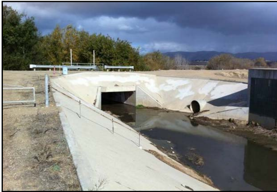
Figure 2.2-3. Santa Maria Levee Box Culvert Where Unit 2 Flows into Santa Maria River (looking northward)
