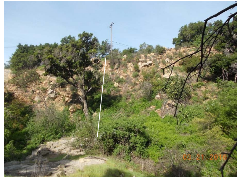
d. Slope storm drain alignment, power pole to rock rip-rap in foreground
