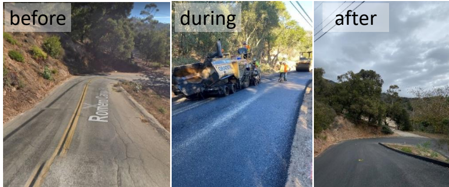
Romero Canyon- SCE settlement funding
