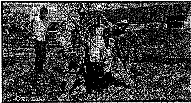
Power Corps members help install and maintain green stormwater infrastructure in Philadelphia. Power Corps supports youth workforce development and environmental stewardship and resilience. Photo Credit: Philadelphia Water Department.
