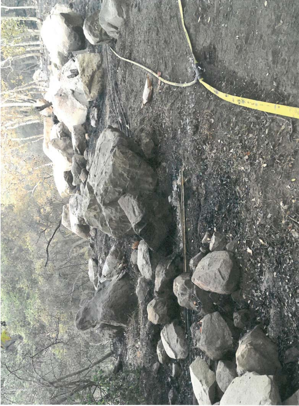
6. 949 Toro Canyon access road 12/14/17. East embankment above creek, hoses and burned area.
