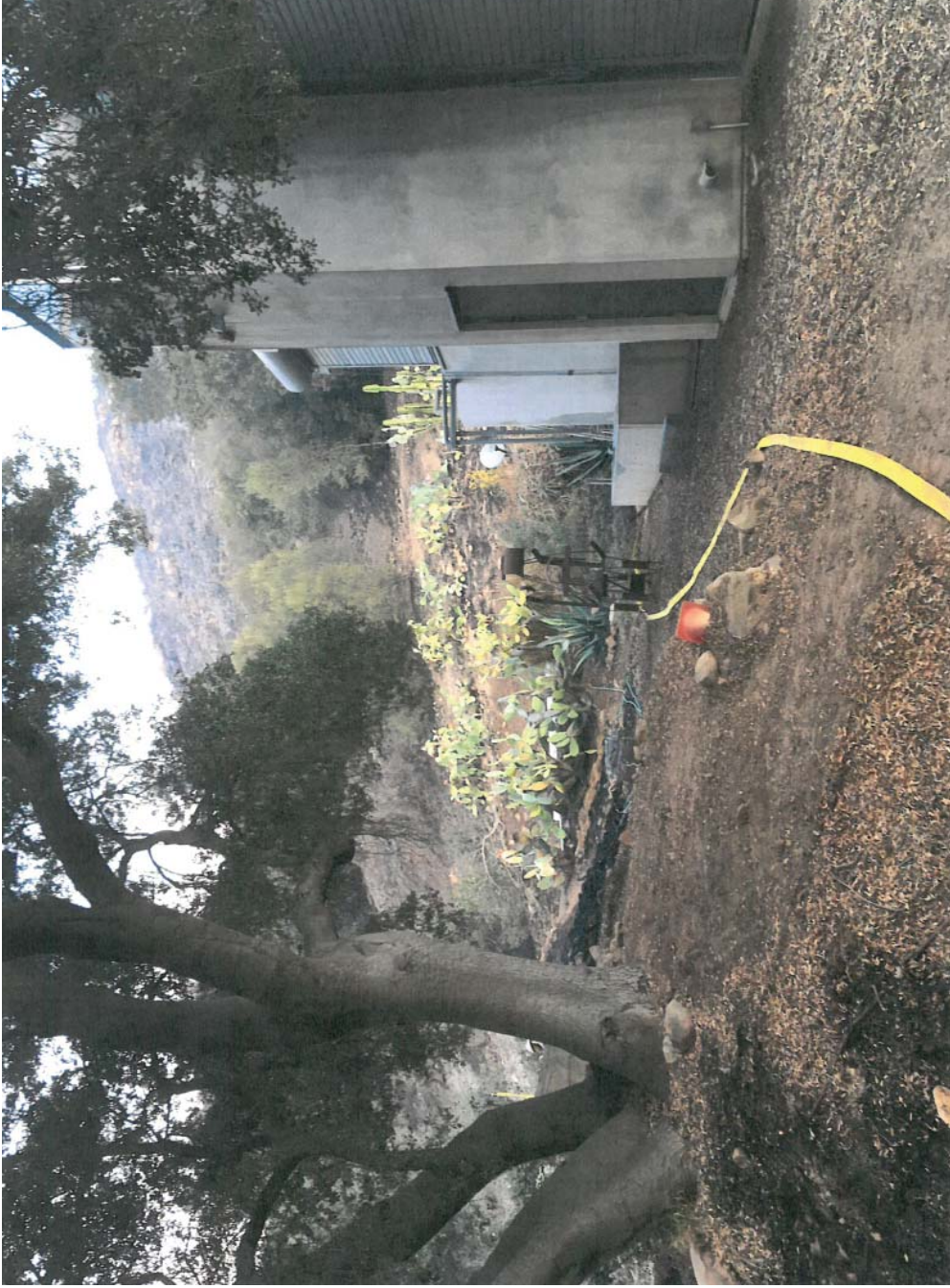
8. View of fire hose west of accessory building. Fire burned within 10 feet of the building.
