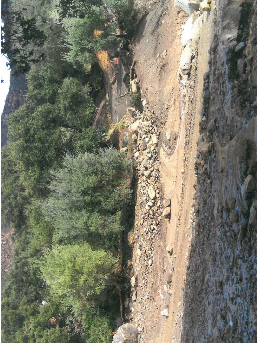
13. Easement road blockage view east. 1/9/18.
