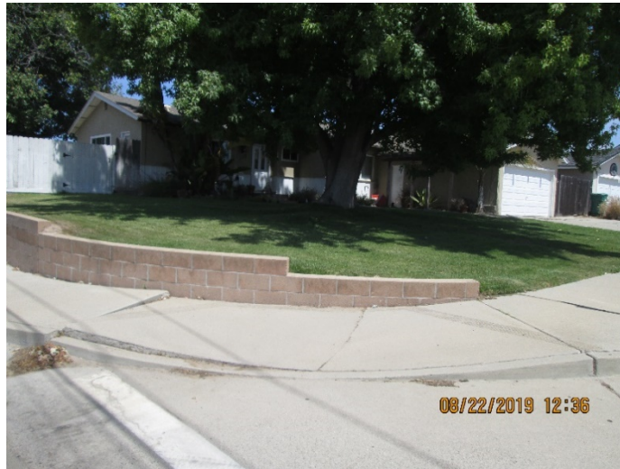
Intersection at Orcutt & Eileen- damaged curb ramp.
