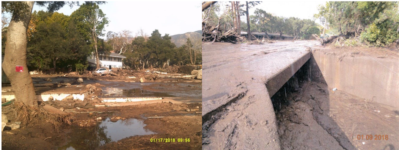
Hot Springs Road, County Bridge 51C-41: 1) Debris flow entered roadway and shoulder, damaging and destroying AC dike, drainage inlets, and traffic control signs. 2) Approach and bridge barrier washed away by debris overflow.
