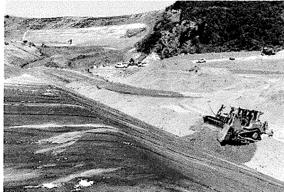
A dozer pushing protective cover soil up a lined slope at Tajiguas
