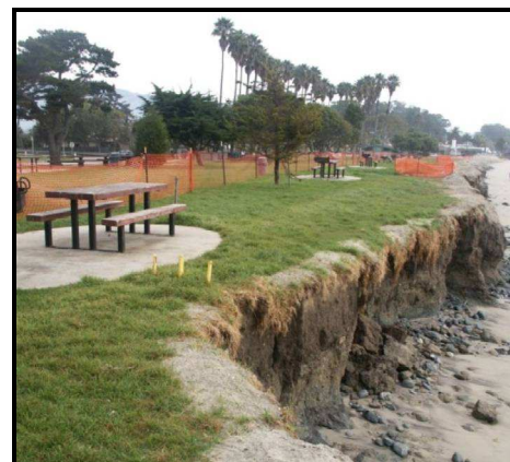
Family Picnic Tables and adjacent storm damage
