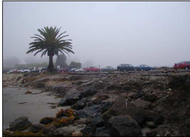
Storm wave action – 34 parking spaces have been lost
